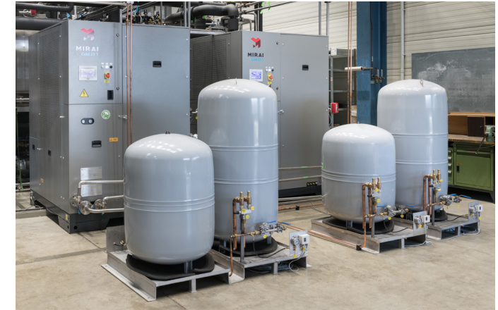
A contained ethane/propane cascade cooling system.
